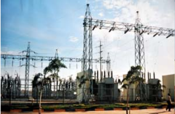
Khmer Power Plant at Mean Chey district
